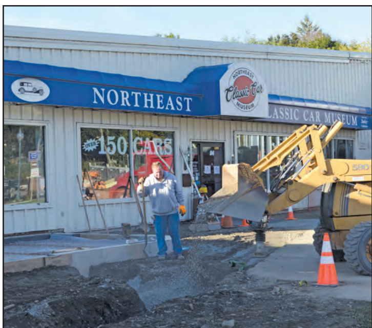
In the fall construction began on the Norwich Museum District including new sidewalks in front of the NECCM. (Photo by Sarah Genter)
